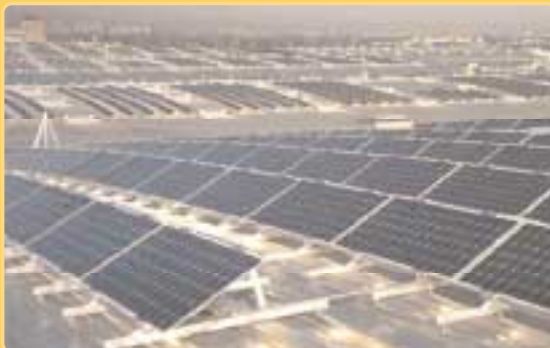
Munich Trade Fair rooftop array 1MWp
