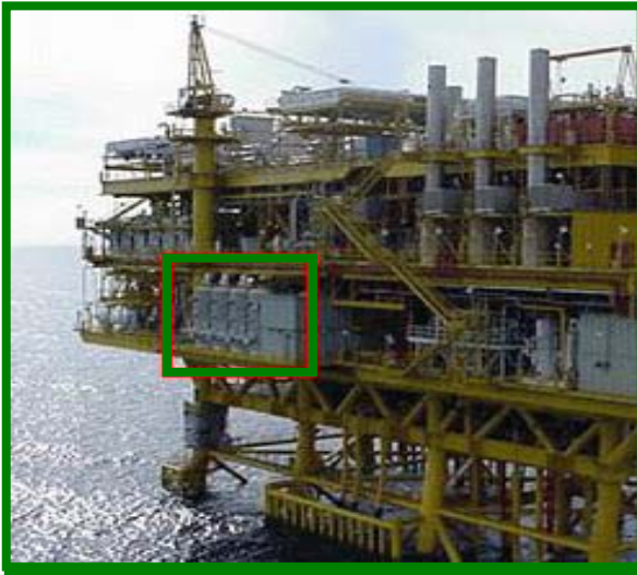
A CO 2 -membrane stripping unit (high-lighted) is attached to an offshore platform operated by Unocal in the Gulf of Thailand. The unit shown here is handling 1.8 mt CO 2 /yr.
