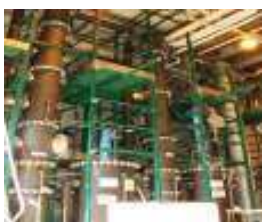
Alstom Labs Växjö Sweden - 0.25 MWth Post C. - multi purpose
