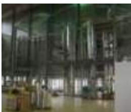
EoN Karlshamn Sweden - 5 MWth Chilled Ammonia-Fuel oil
